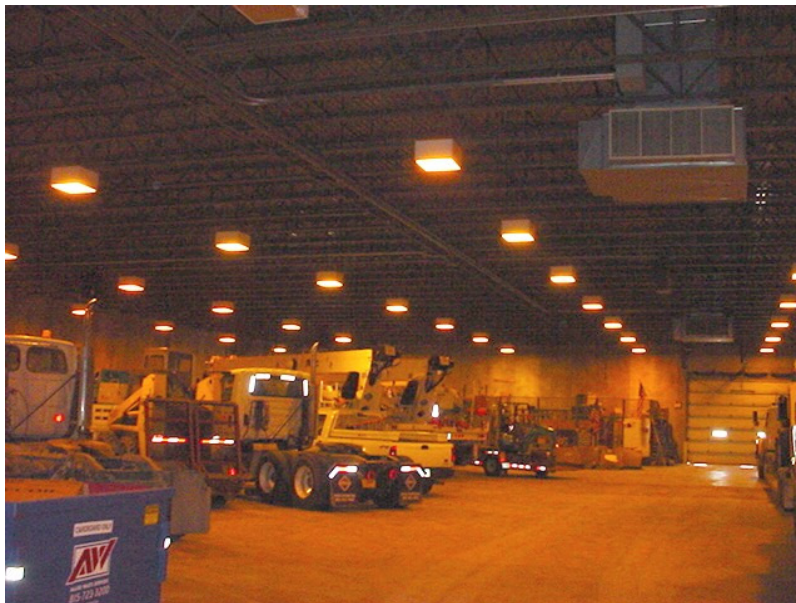
Existing Lighting System: (45) HPS fixtures, 300 W/ea.
